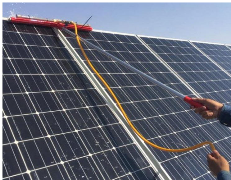
Manual wet cleaning of modules at AEP-I's solar PV plant in Ma'an First Solar Park with hand-held water brush
