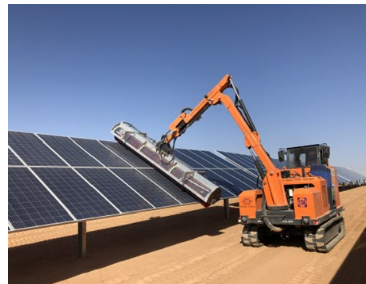
Dry-cleaning of modules at AEP-I's solar PV plants in Benban Solar Park with a BP Solar Cleaner F3500 C-AP
